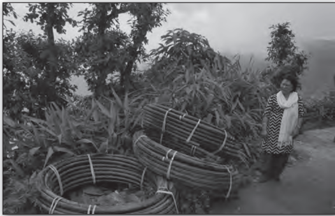
Water supply pipes for Bhattedanda.
